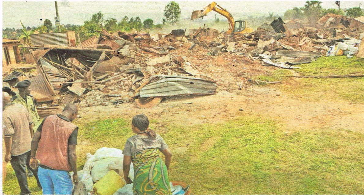
People look on as a tractor demolishes their houses in Lubigi wetland last week. PHOTO/NOELINE NABUKENYA
