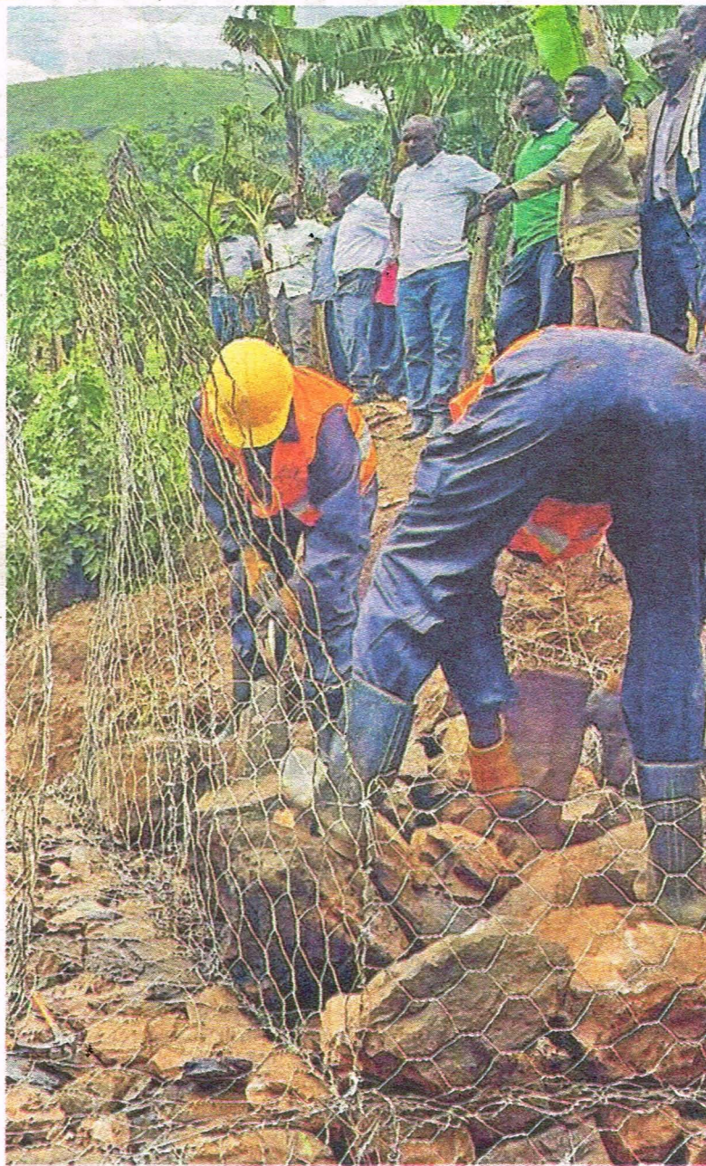
Resident look on as gabions are constructed to stop soil erosion in Muhito, Sheem District. PHOTO/ MONITOR
